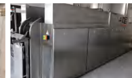
盐城高新区伍佑垃圾处理站 Wuyou Garbage Disposal Station in Yancheng High-tech Zone
