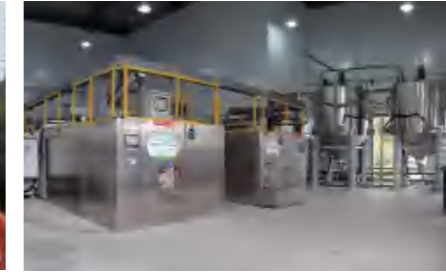
南京江宁开发区垃圾中转站 Nanjing Jiangning Development Zone Garbage transfer Station Capacity/处理量：15t/日(d)
