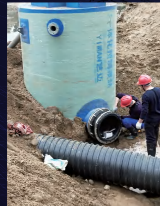
PPP project of sewage treatment for villages and towns in Honggan County MODEL: YMPS-300-5.3-2-S
