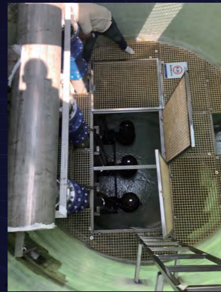
Zhujiajiao Town rural domestic sewage Treatment project MODEL: YMPS-120-4.55-2-S
